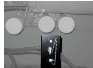
Battery switch on bracket
