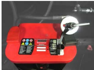
Battery switch mounted on the battery itself
